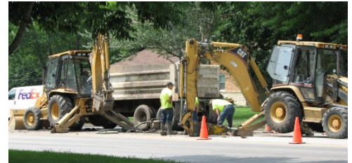
BEWARE STRUCK-BY HAZARDS LIKE TRAFFIC, SWINGING BACKHOE BUCKETS OR DROPPED PIPE.
